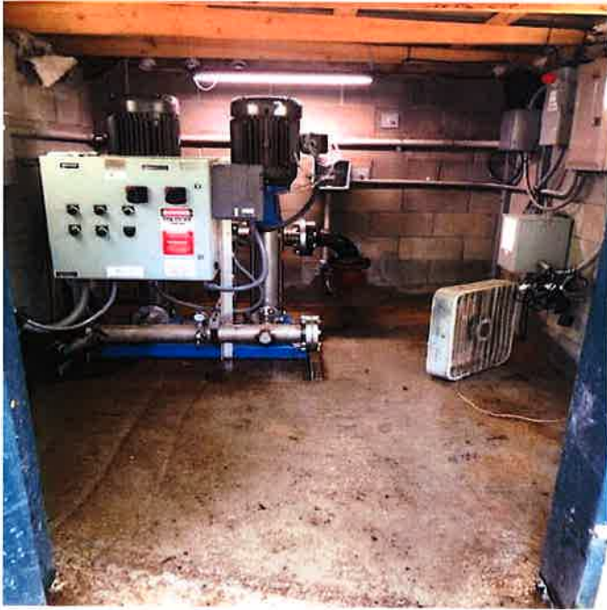
Pictures now show that all wires have been removed that were UN needed and the building clean.
