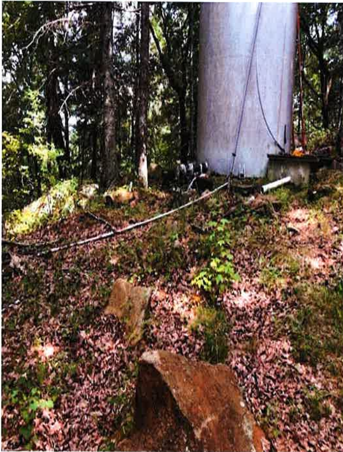
Again this picture shows wires are laying everywhere along with trash and debris.
