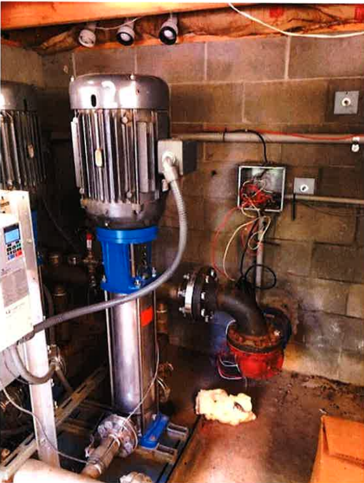
Original Inspection report shows wires hanging out of boxes coming into the building from the outside elements.
