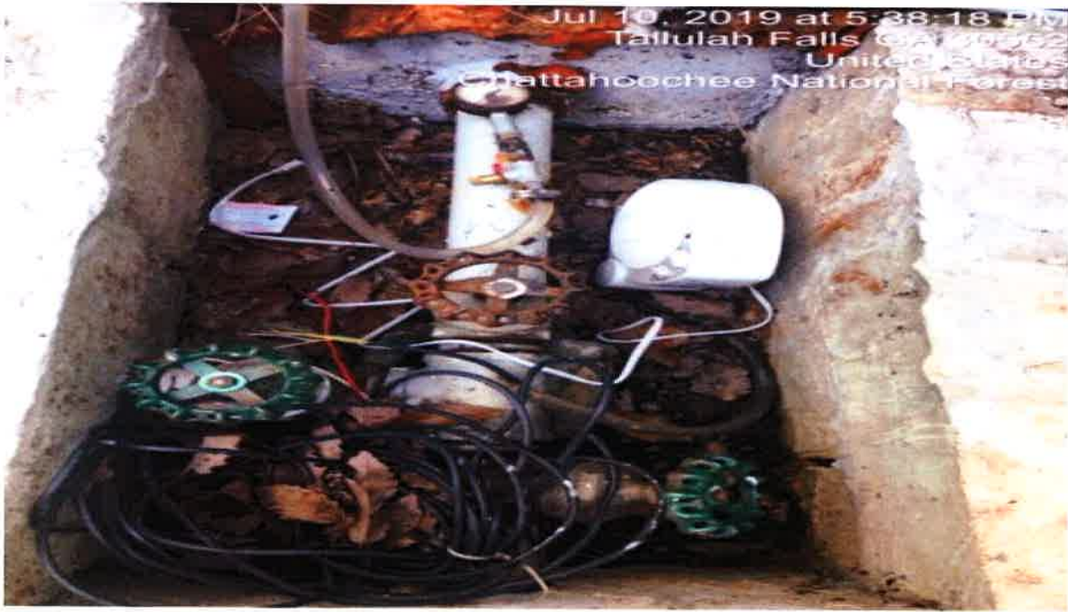
Heavy rust around the discharge pipe of the tank and valves that control flow.
