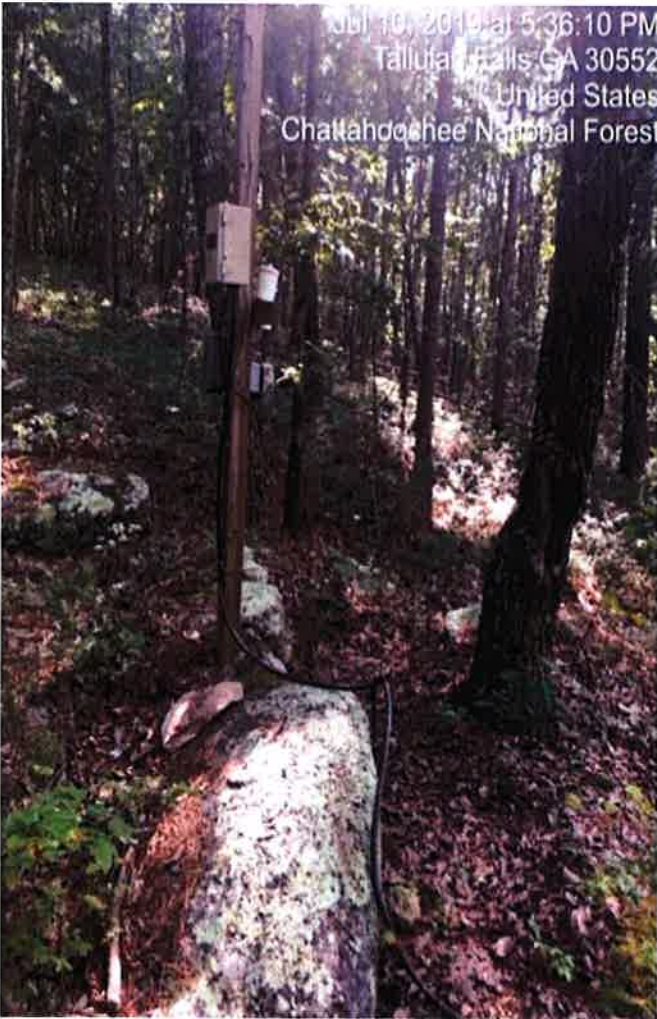
Exposed wires and controls that are open to tampering, this will have to be made safe.
