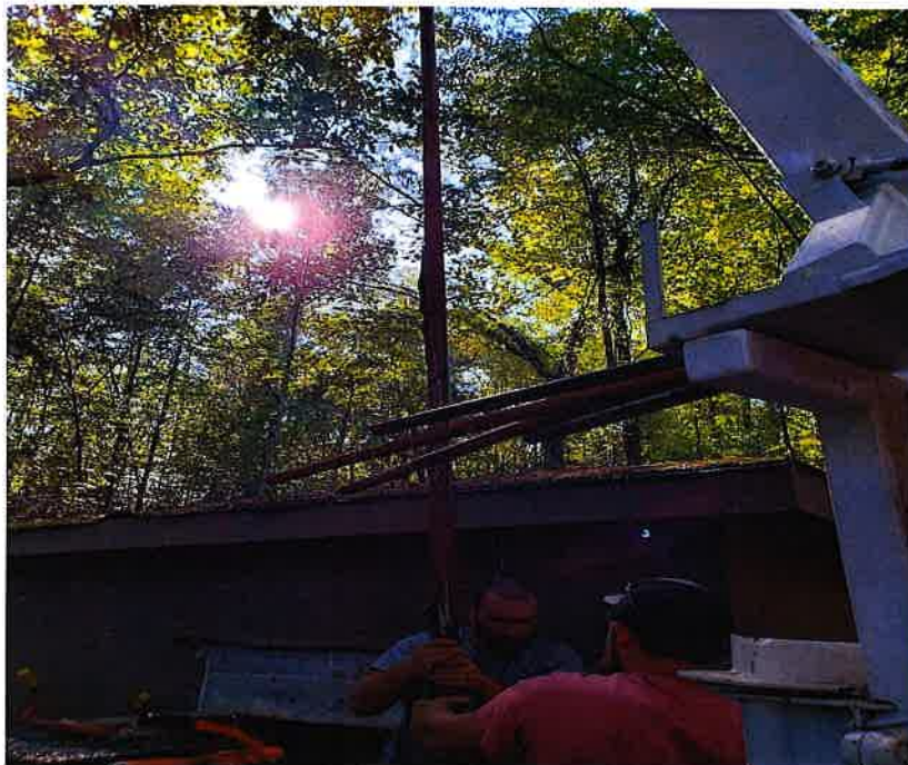
Pump being removed and pipes stacked as you can see on the pictures there is a lot of Iron Sludge attached to the piping.
