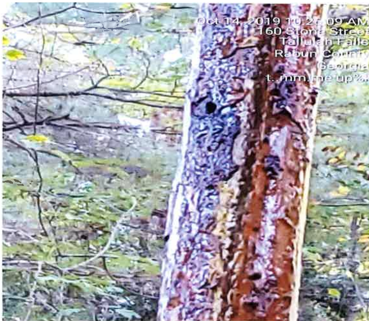
This is the discharge pipe for the well pump, as you can see there is 1 prevalent hole in the line with many small included. Again the line is covered in Iron sludge from the well.
