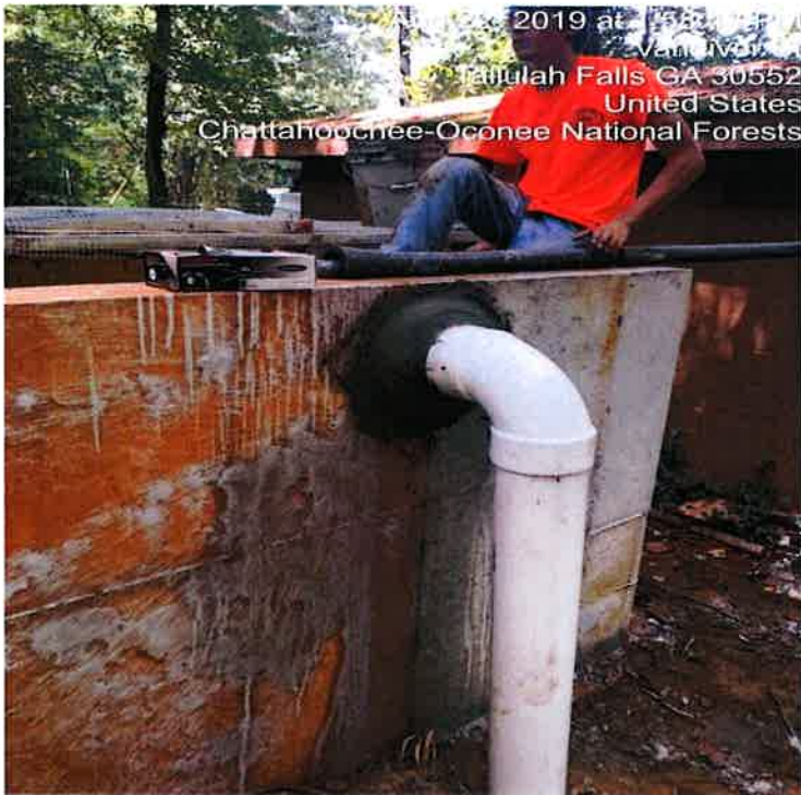
Picture 3. Pipe through the wall for the overflow has been grouted and sealed in with Hydraulic cement.
