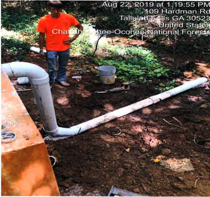
Picture 2. Pipe has been installed and connected to the current drain line.
