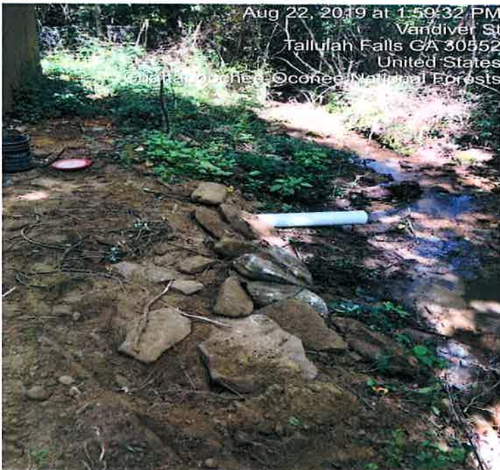
Picture 7. River bank has been cleaned up and left over stones placed for erosion purposes.
